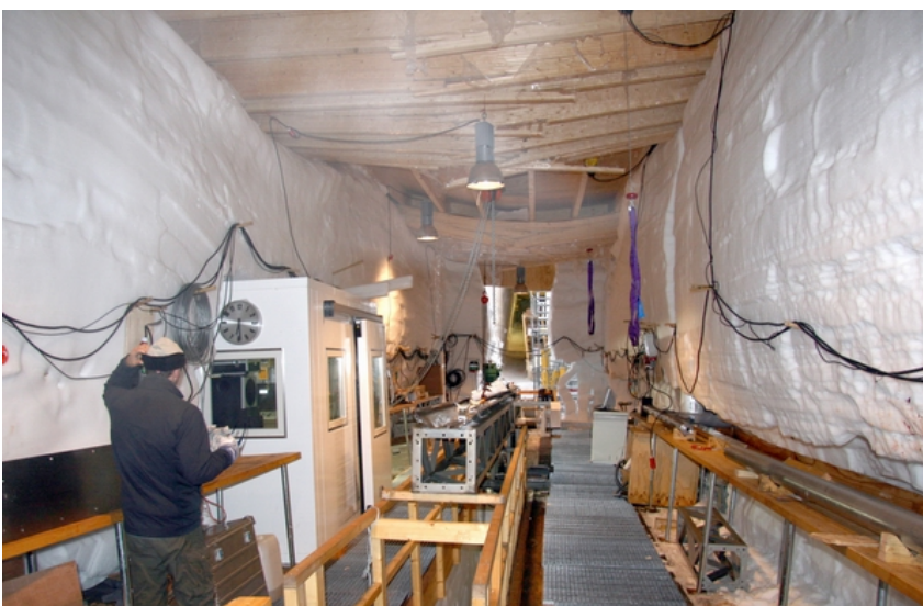
NEEM drill trench in 2012. Note the broken beams.
