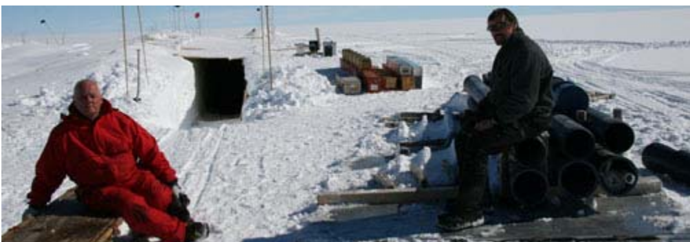
Camp activities: snow blowing and moving the heavy casing tubes down into the drill trench.
