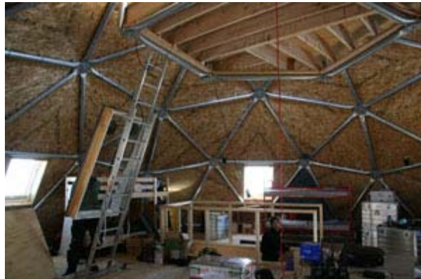
Dragging the last top window up the ladder to the pentagon in the top of the dome.
