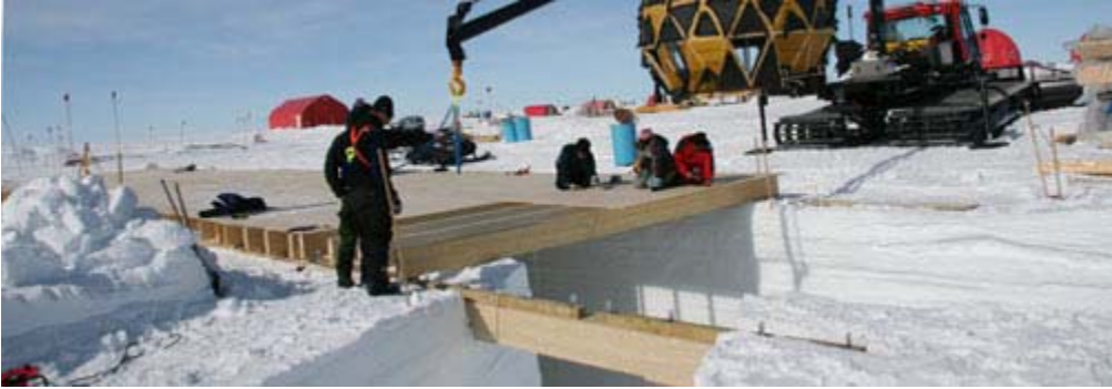
Construction of the bridge part of the roof. Peter is secured to the crane.
