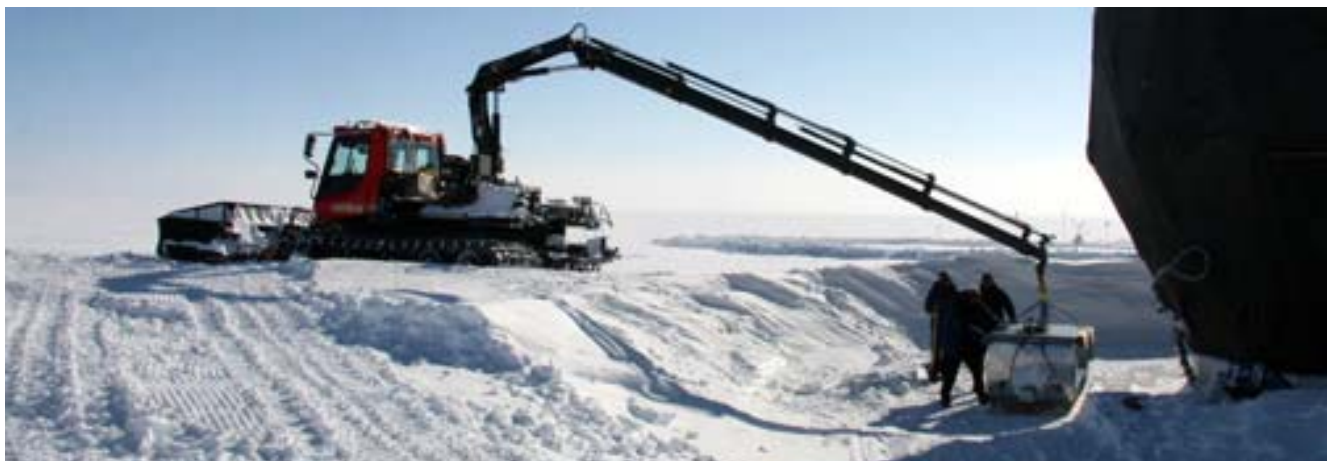
The rebuilt main snow melter is put in place next to the main dome..
