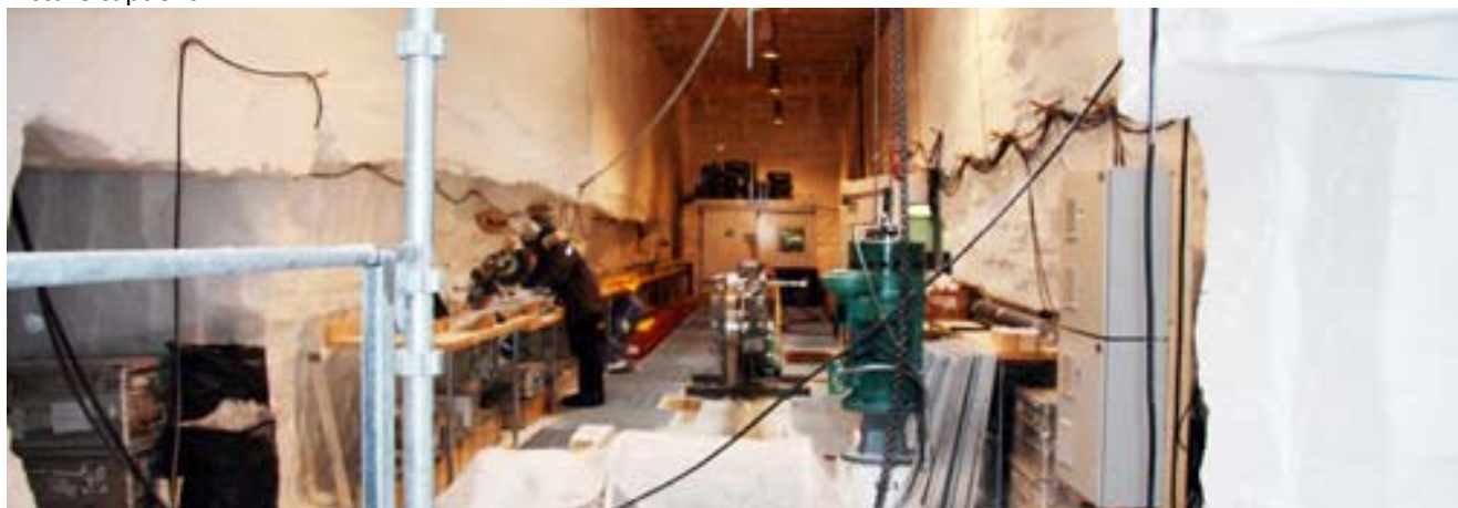
A new view into the drill trench from the staircase (the rods to the left).
