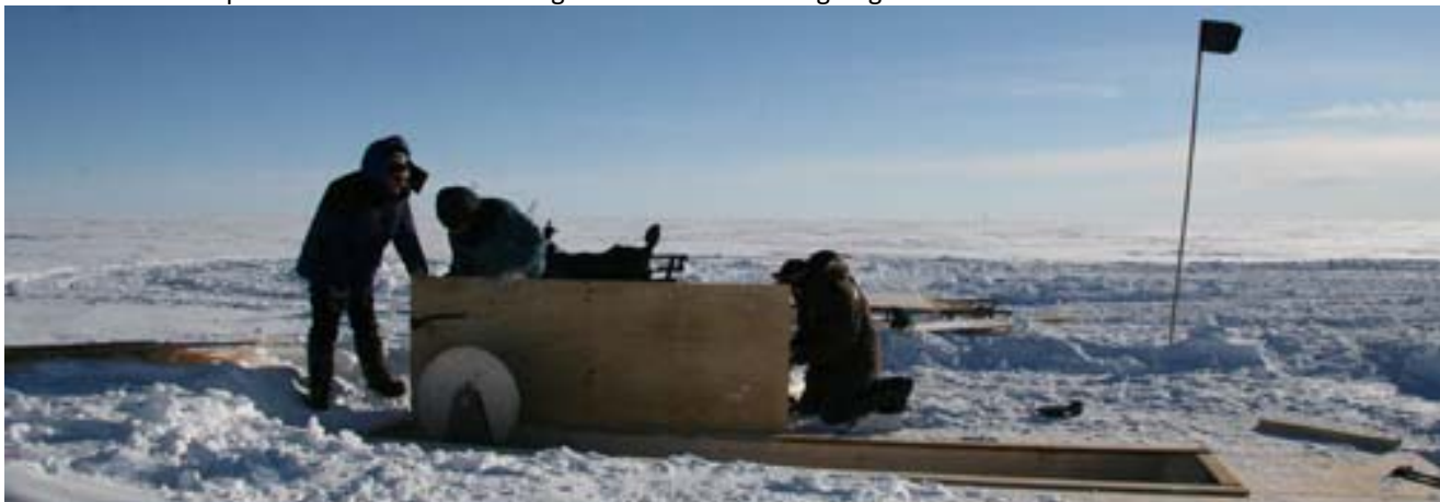
Sverrir, Oli and Hans Christian mount sections of "the submarine" skylight on the drill trench roof. To the left, the top wheel, or sheave of the drill tower can be seen pointing up from below.
