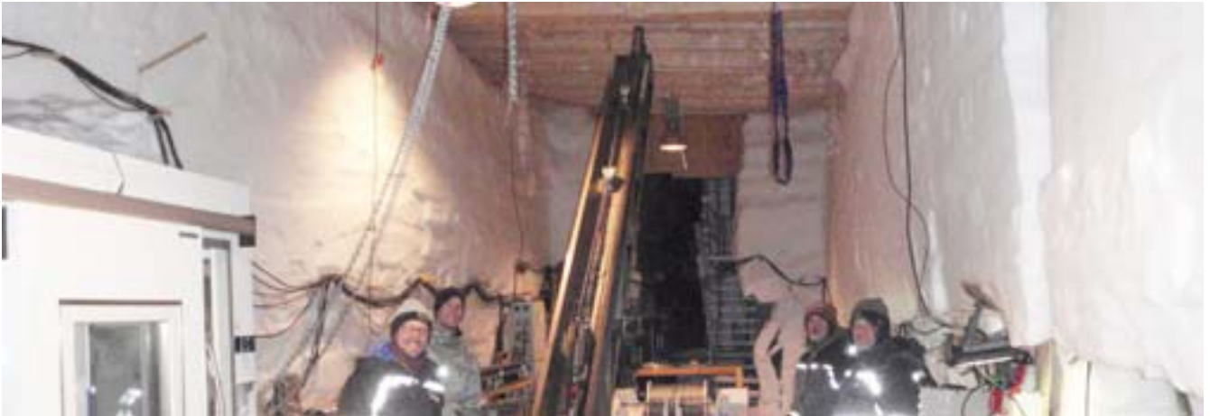
Tower: Top of the tower touches the roof beam before shortening. From left to right: Trevor, Simon, Bruce and Carsten.
