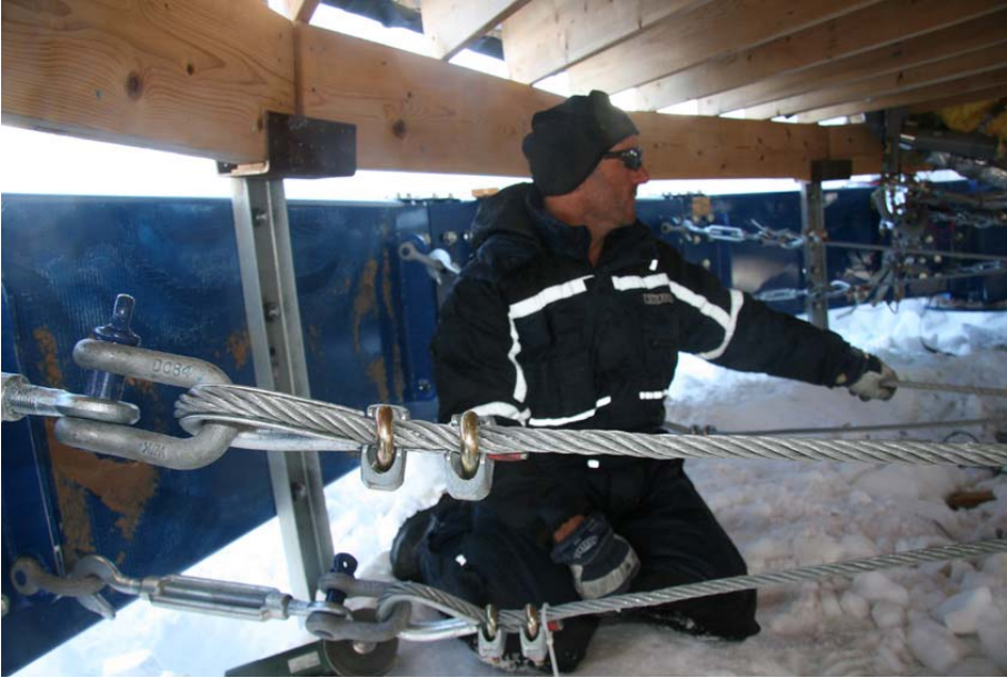
Villi adjusting the cables under the Dome
