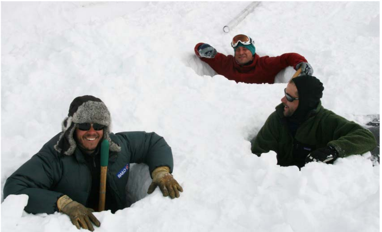
Frogs in the holes ... Drilling the holes for the legs of the solar panels D-frames
