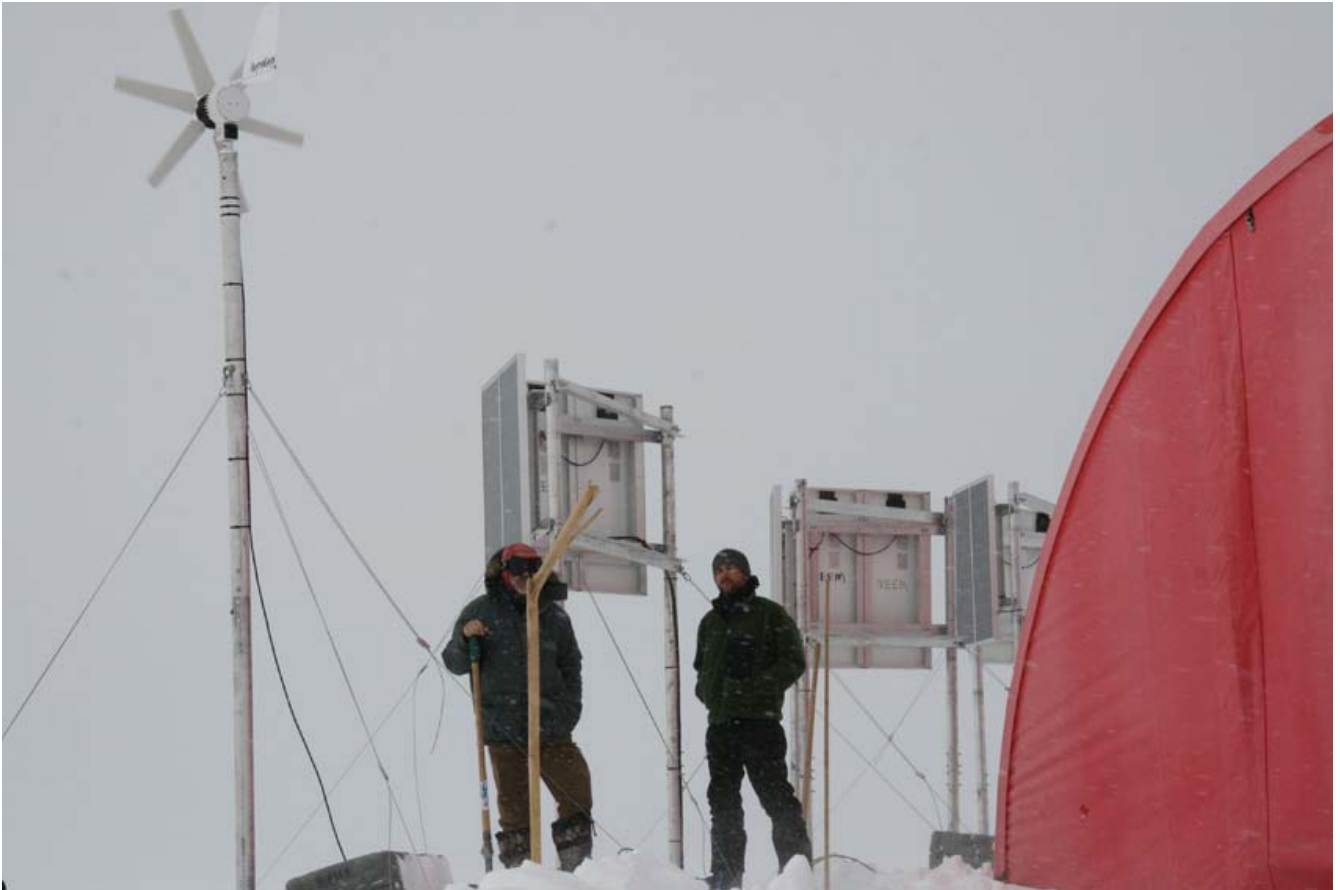
GLISN solar panels and wind turbine installed
