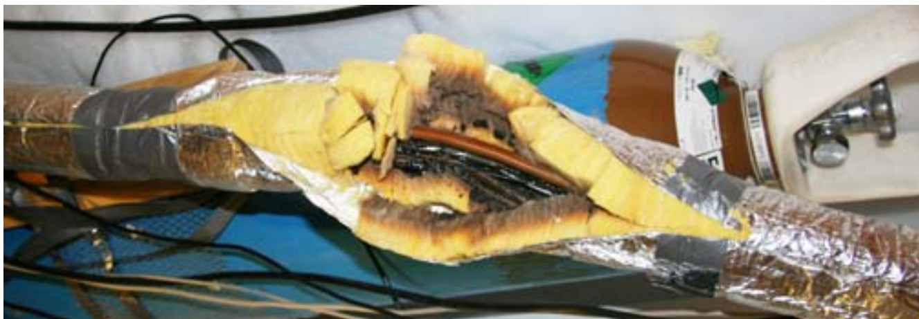
The connection lines between the CFA and GIL labs appear to have been sufficiently heated
