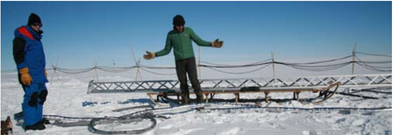
Building the tower for the water vapour program and finding all the tubes to attach to the tower. Hans Christian (on picture) and Fredrik have Scott (on picture) as helper until the basal ice drilling program starts in few days.
